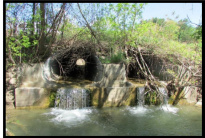
Culverts such as this these can constrict the natural flow of the stream, have a perched outlet that only strong swimmers can jump and contain no natural streambed. Many culverts and dams fragment
